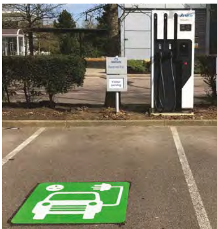
Above: Electric vehicle charging point – Hatfield, UK One of 12 new electric vehicle charging points installed at our Hatfield offices.
