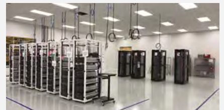
Below and bottom right: Integration Center – Livermore, California In 2020 we opened a major new facility next to Silicon Valley, close to major hyperscale customers.
